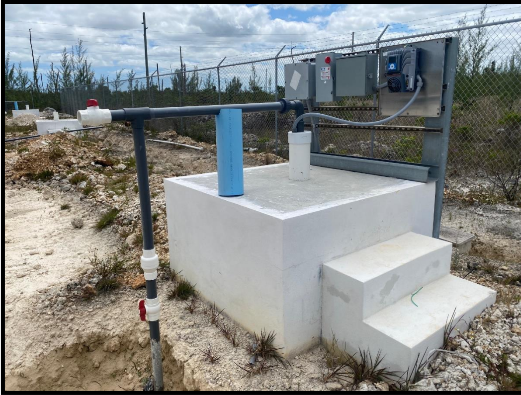
Figure 163. Operational Well. Source: PlanEHS, 2024.
