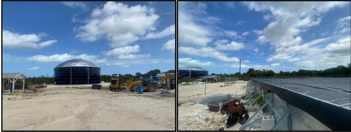
Figure 156. Treated water accumulation tanks: (a) New 1,000,000-gallon tank; (b) Collapsible tank. Source: PlanEHS, 2024.
