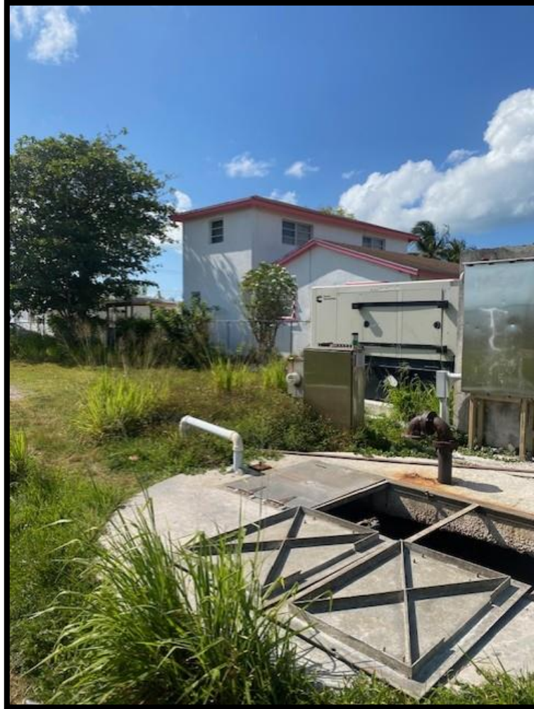
Figure 19. Well Chamber, Pump Control Panel, ventilation, and Power Generator in Elizabeth East LS. Source: PlanEHS, 2024
