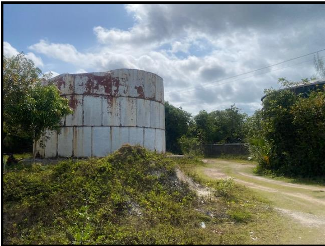
Figure 157. Unused Damaged tank. Source: PlanEHS, 2024.
