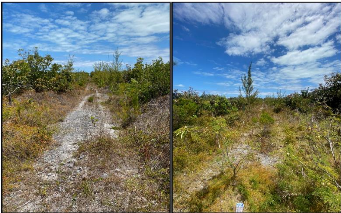
Figure 112. Uncleared and unpaved roads. Source: PlanEHS, 2024.
