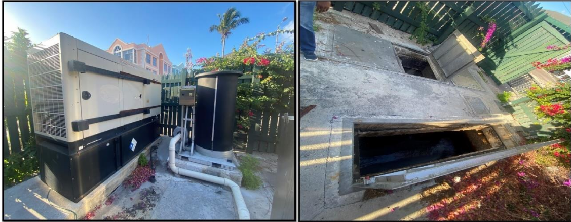
Figure 138. Rawson Square Lift Station: (a) power generator and Chlorination Dosing Machine; (b) well chambers. Source: PlanEHS, 2024.
