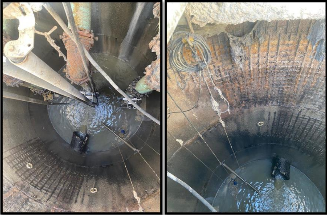
Figure 21. Well Chamber of Elizabeth East LS. Source: PlanEHS, 2024.
