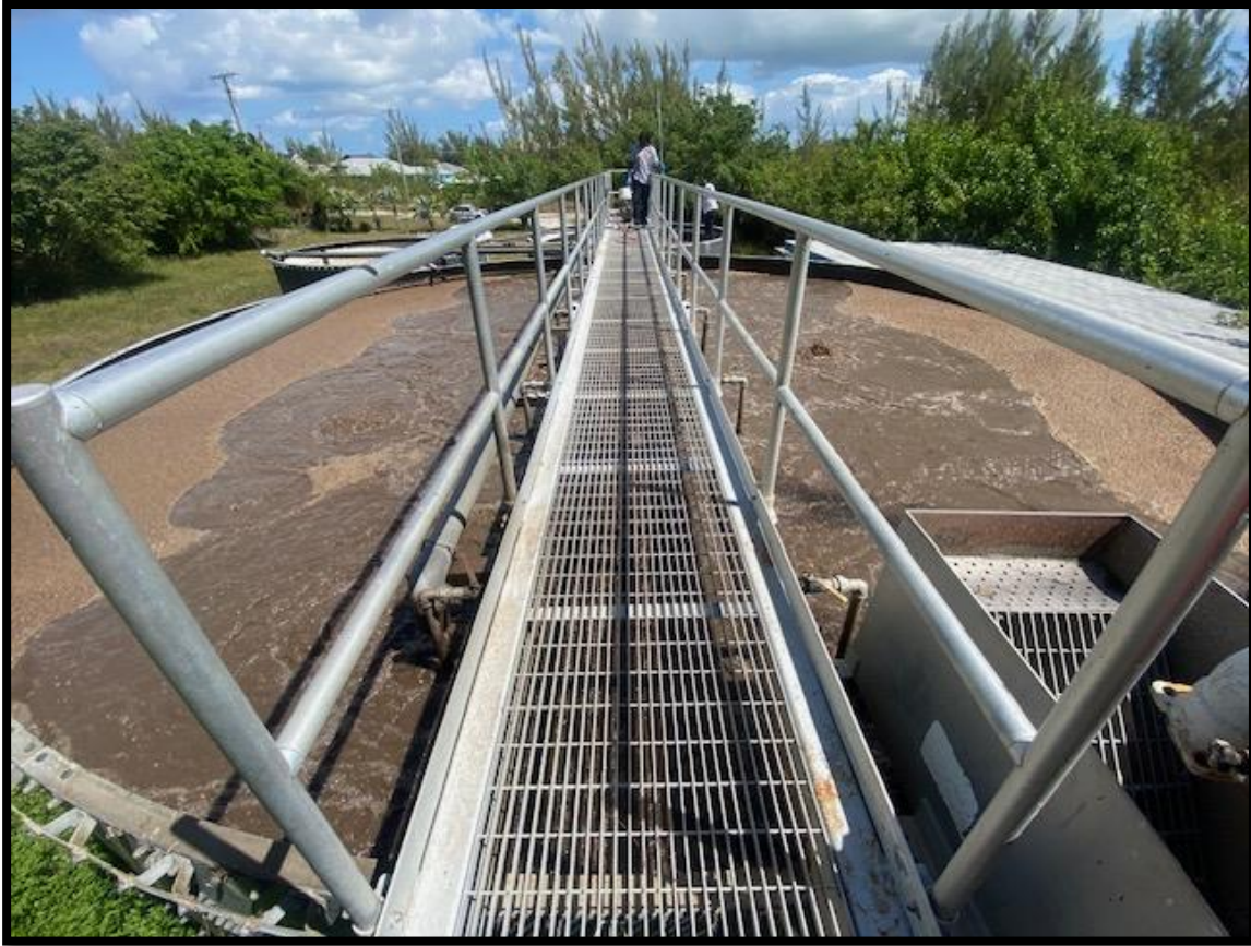
Figure 168. Aeration tank with grid for solid removal (right). Source: PlanEHS, 2024.
