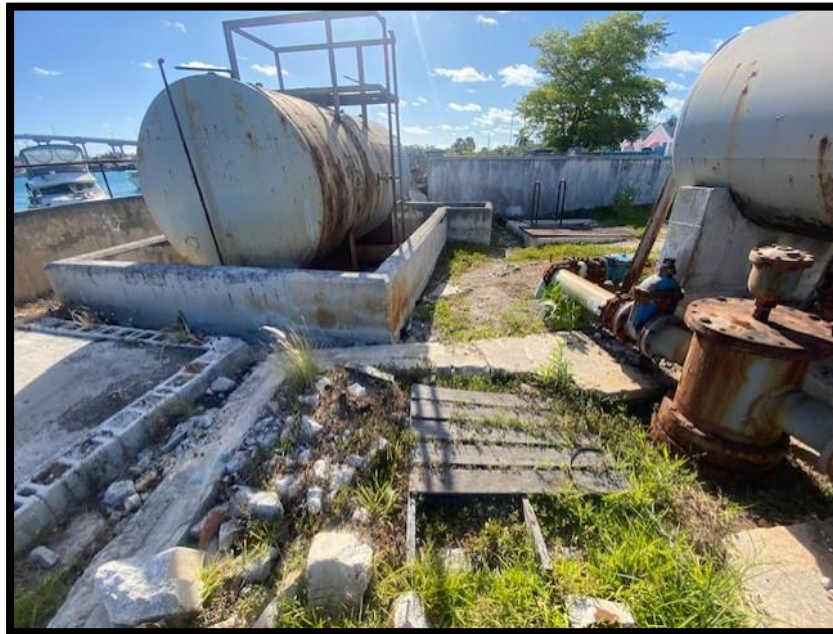
Figure 143. Unused fuel tanks that need to be removed from the premises. Source: PlanEHS, 2024.
