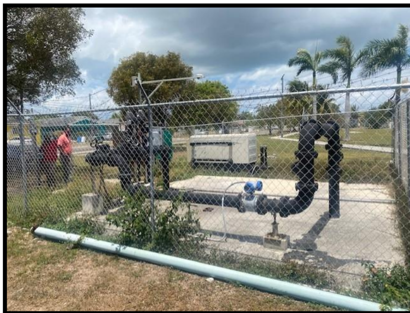
Figure 14. Flamingo C Lift Station. Source: PlanEHS, 2024
