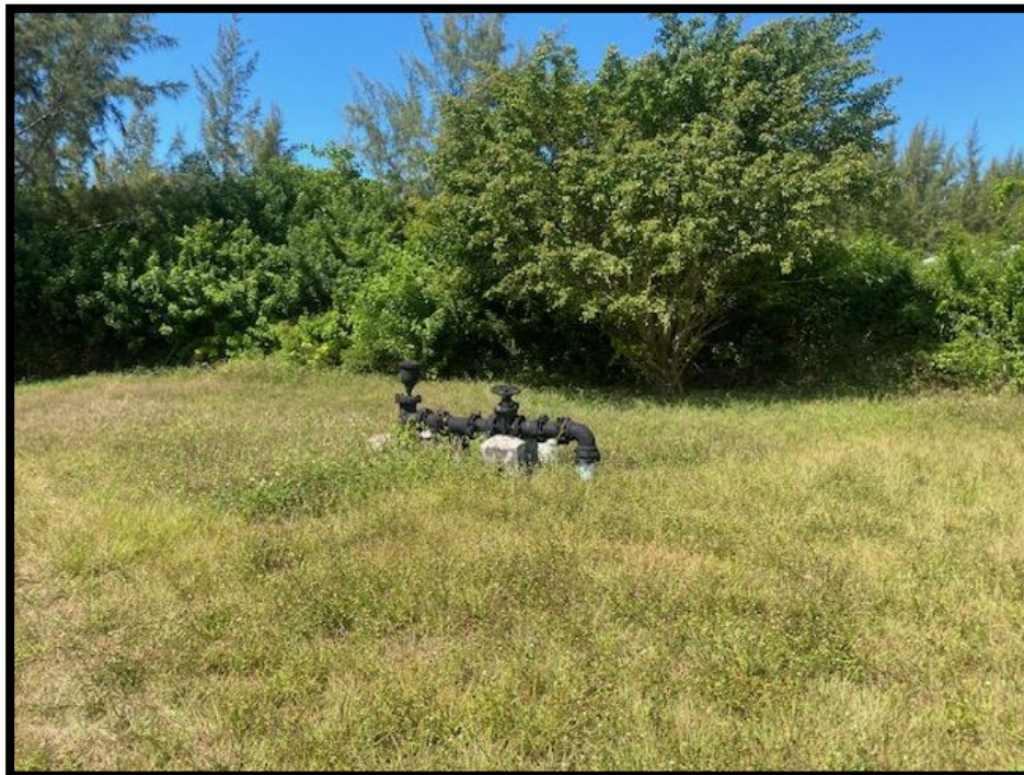
Figure 170. Injection well for treated wastewater. Source: PlanEHS, 2024.
