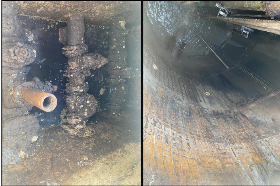
Figure 131. Elizabeth East Lift Station conditions: (a) rusted valves in valve chamber; (b) severe deterioration on well chamber. Source: PlanEHS, 2024.
