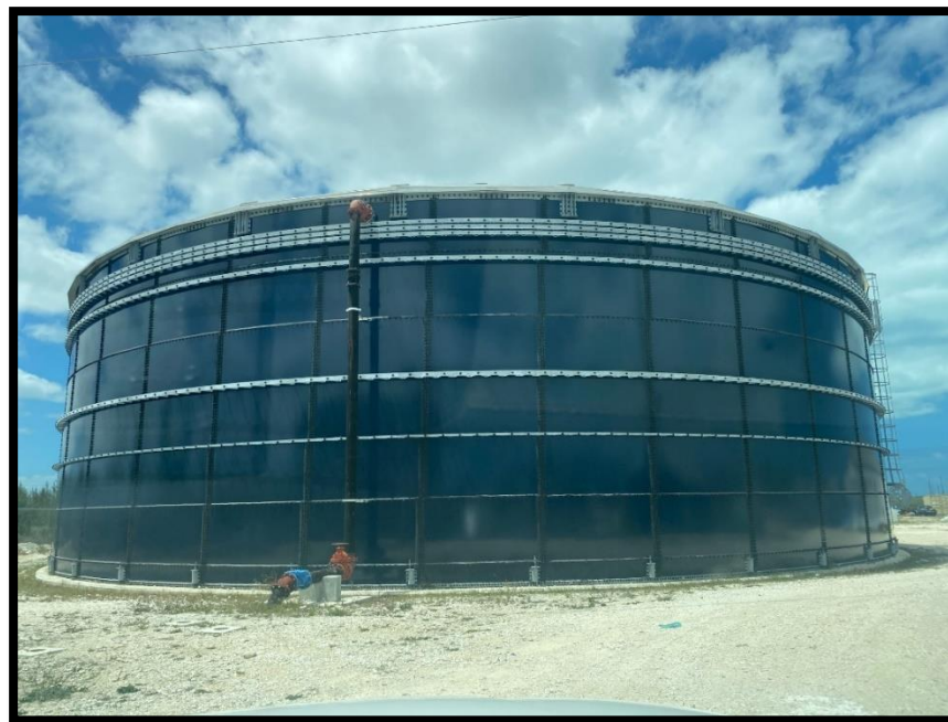
Figure 165. New 1.5 million imperial gallon storage tank. Source: PlanEHS, 2024.
