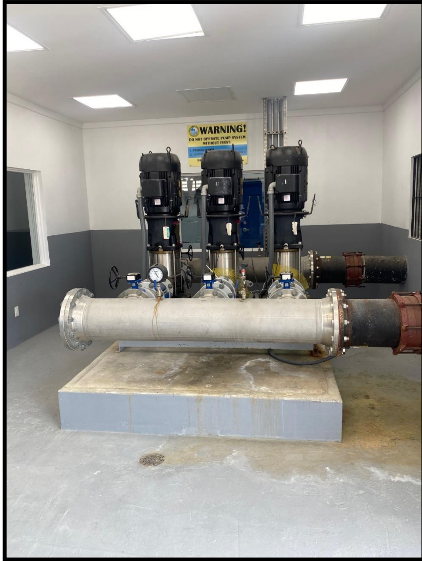
Figure 162. Pumping System at Marsh Harbour Pumping Station. Source: PlanEHS, 2024.
