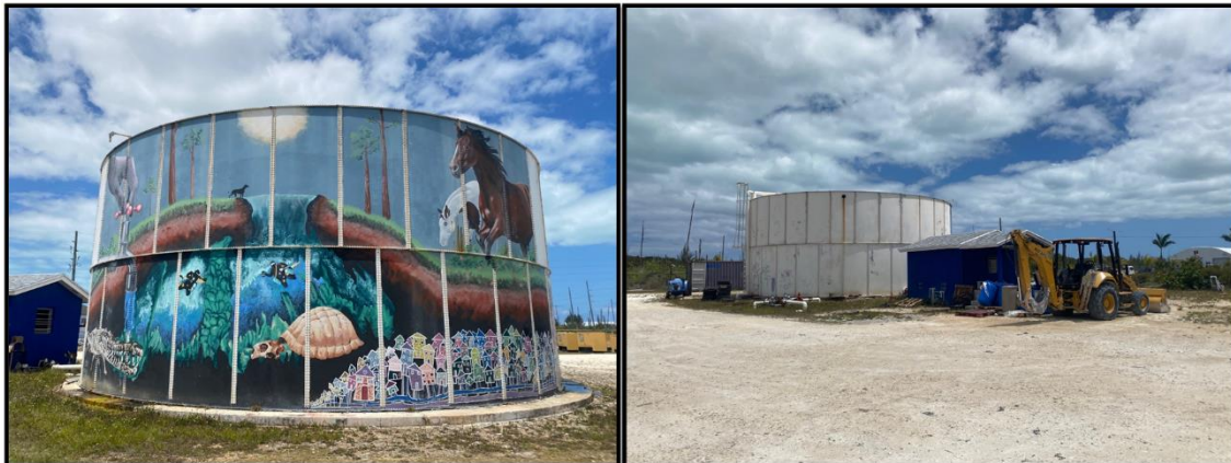
Figure 164. Existing (and damaged) storage tanks at Marsh Harbour Pumping Station. Source: PlanEHS, 2024.
