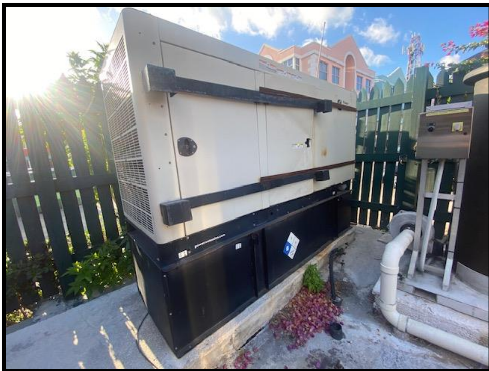
Figure 26. Power Generator. Source: PlanEHS, 2024.
