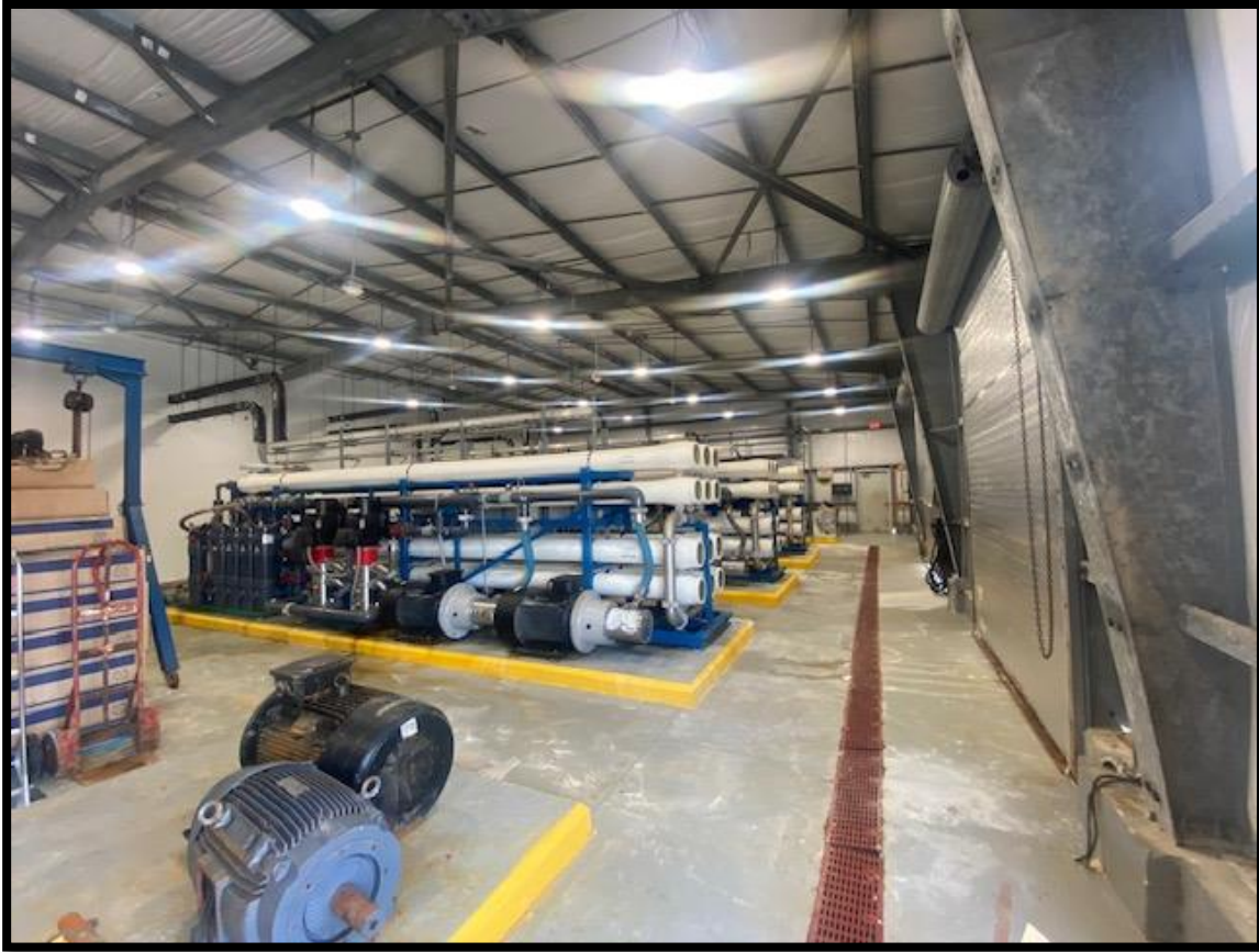
Figure 152. Reverse Osmosis Plant with RO membranes. Source: PlanEHS, 2024.
