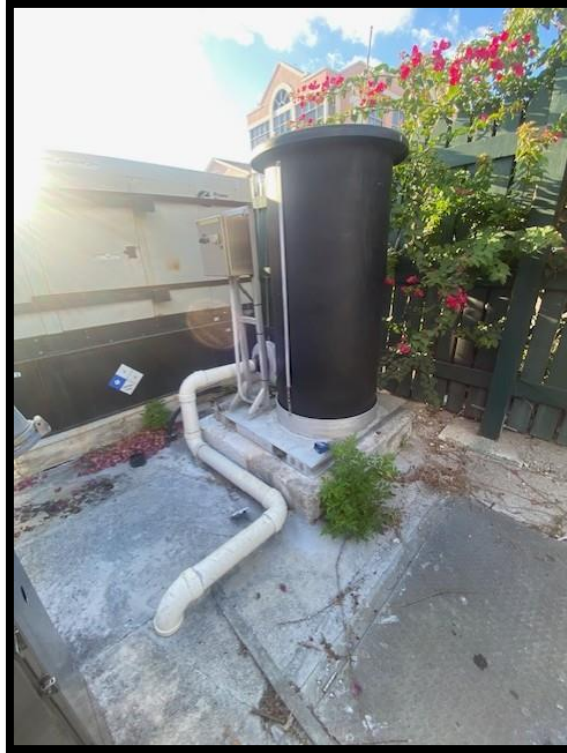
Figure 25. Chlorination station. Source: PlanEHS, 2024.
