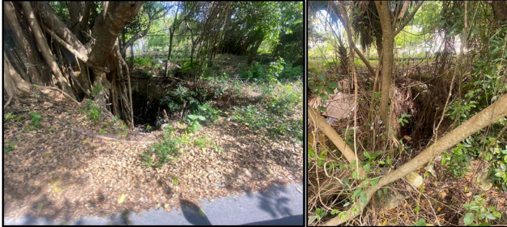
Figure 158. Sinkholes around RO Plant. Source: PlanEHS, 2024.
