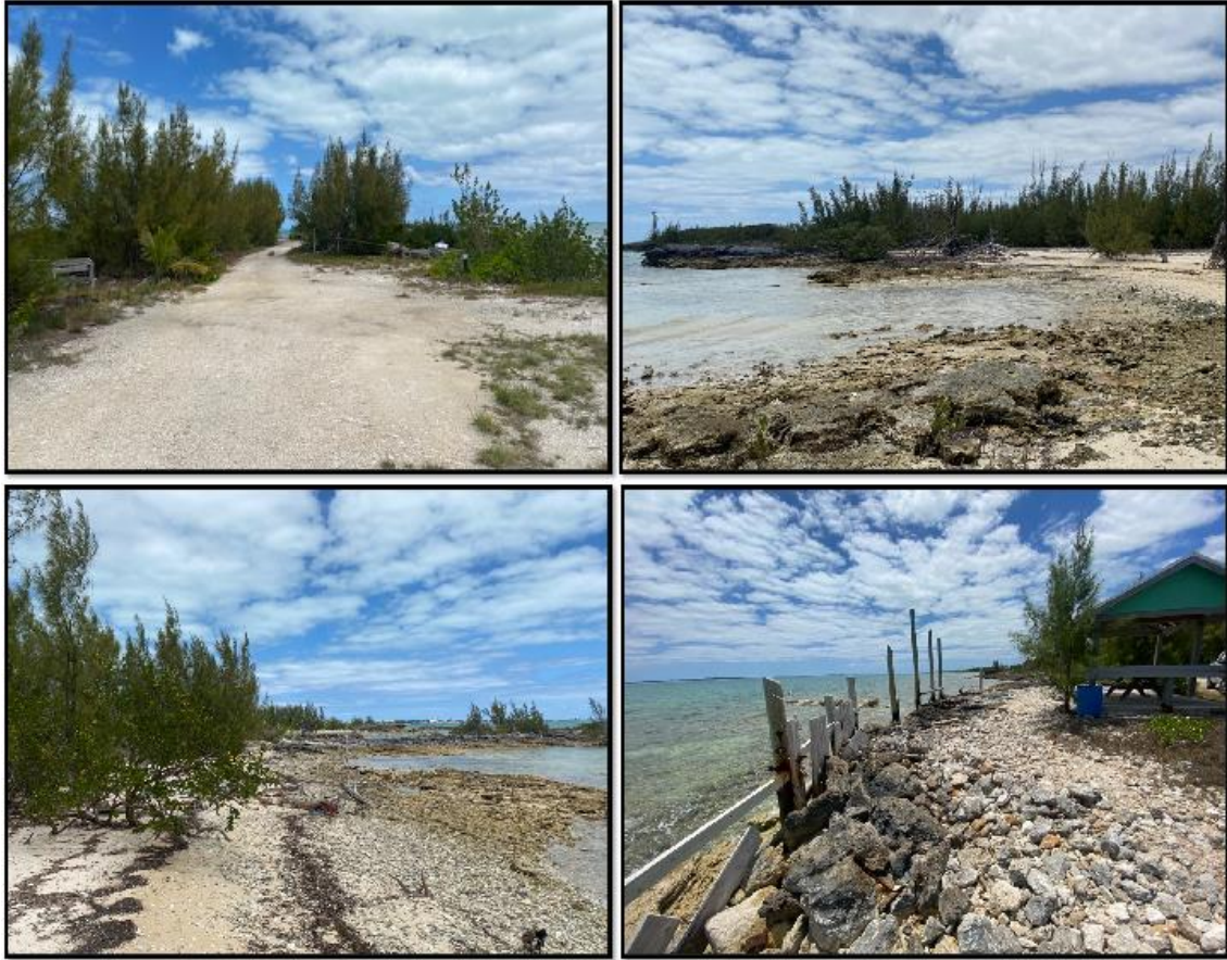
Figure 117. Coastal Area with no seawall and deteriorated wooden balustrade. Source: PlanEHS, 2024.
