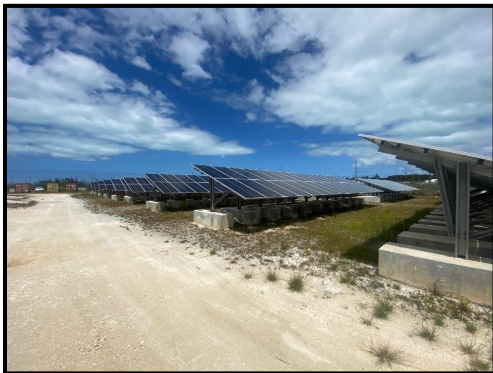
Figure 161. 540 solar panels generating 221KW at Marsh Harbour Pumping Station. Source: PlanEHS, 2024.
