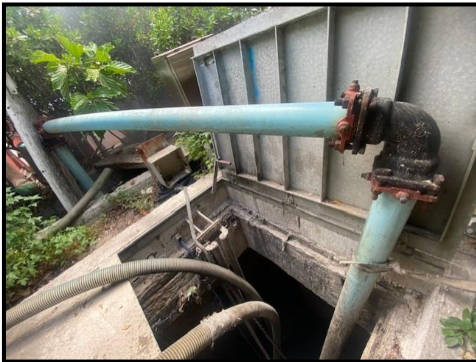
Figure 36. Well chamber and temporary gadget connecting to valve chamber. Source: PlanEHS, 2024.
