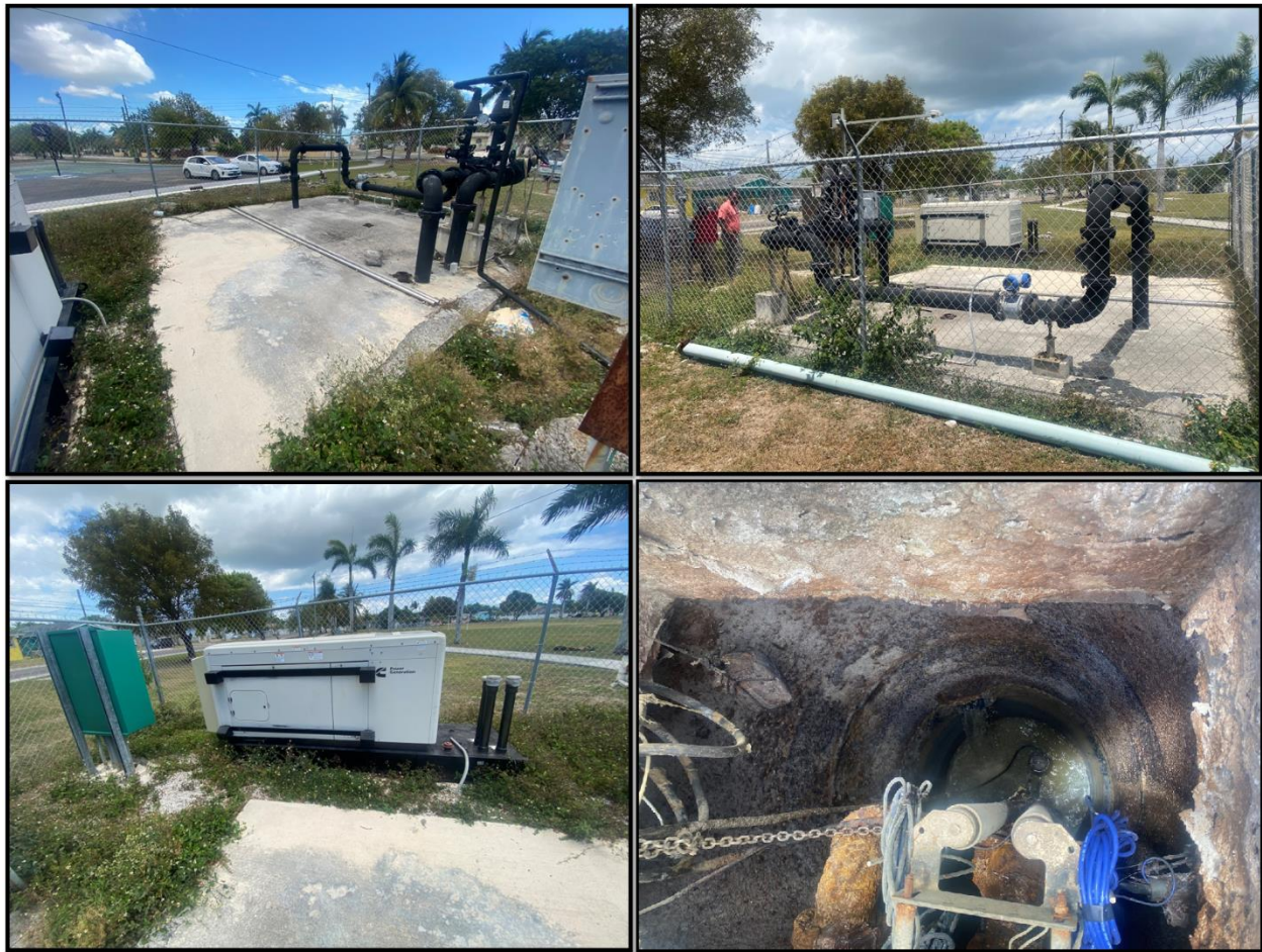
Figure 125. Flamingo C Lift Station: (a) Overground valve system; (b) replaced pipeline; (c) power generator; (d) deteriorated well chamber. Source: PlanEHS, 2024.
