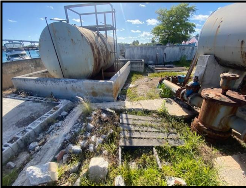
Figure 33. Injection well (right) and unused fuel tank (left) and screening tank (right). Source: PlanEHS, 2024.
