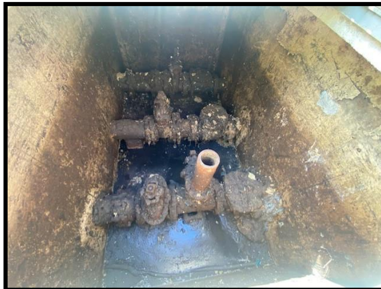
Figure 20. Valve Chamber. Source: PlanEHS, 2024.
