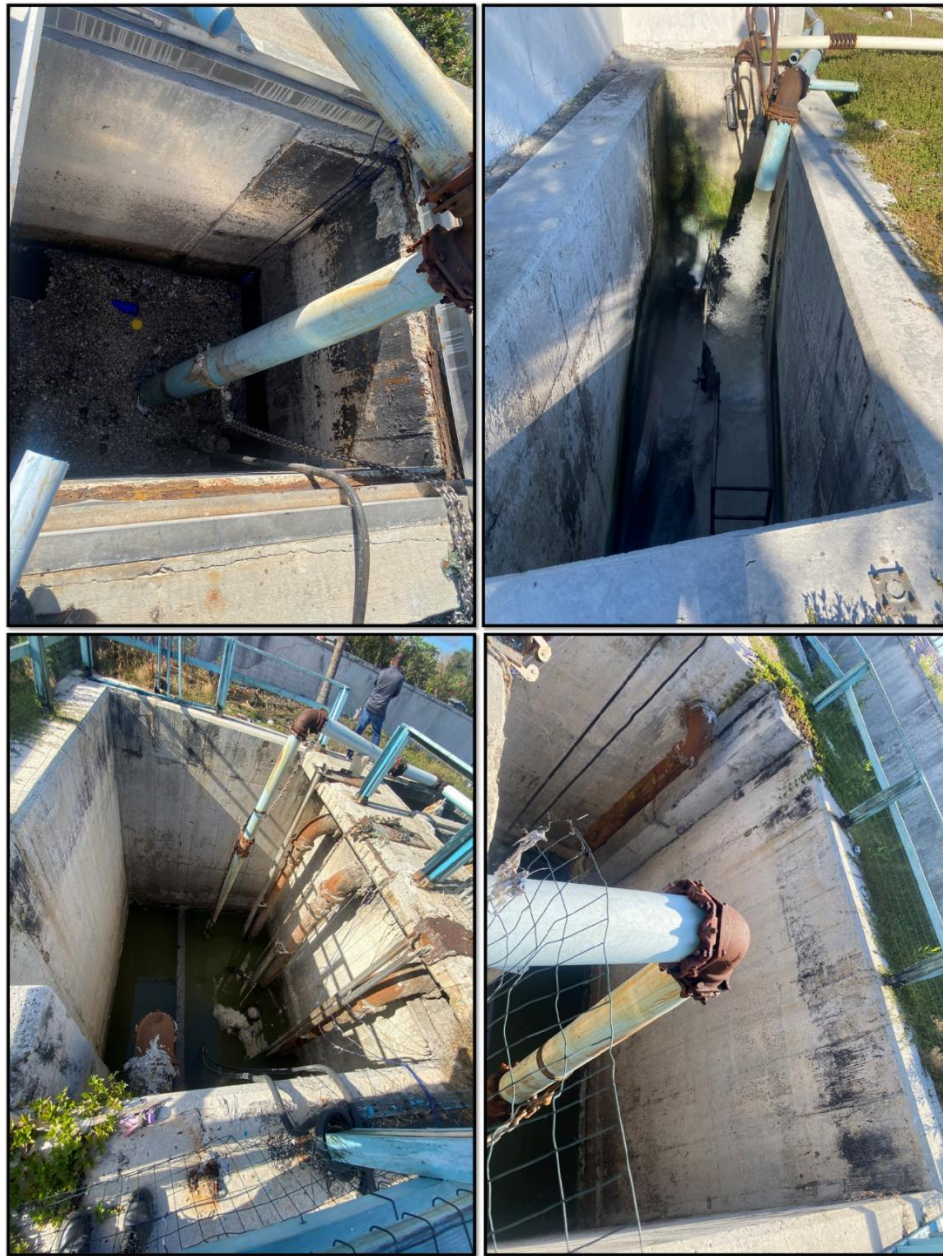
Figure 146. Uncovered well chambers in Malcolm Park Lift Station. Source: PlanEHS, 2024.
