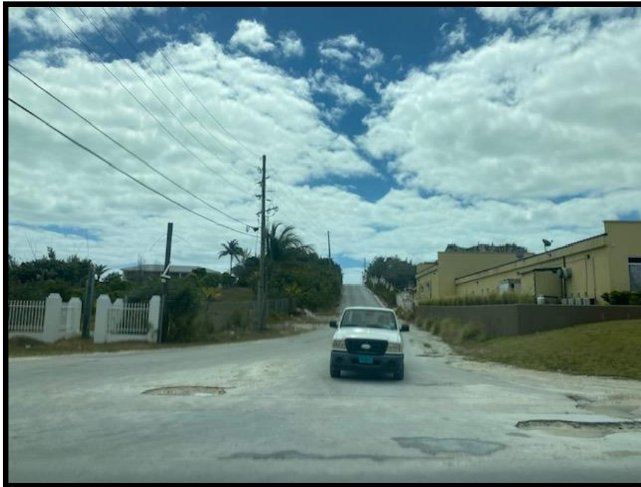
Figure 96. Entrance to Sweetings Tract, Great Abaco Highway and John Sweetings Drive. Source: PlanEHS, 2024.
