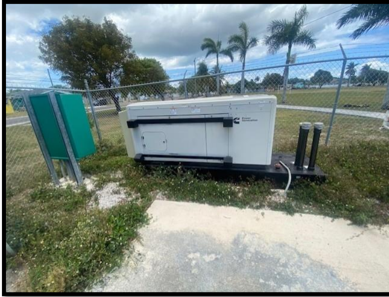
Figure 17. Power Generator. Source: PlanEHS, 2024.
